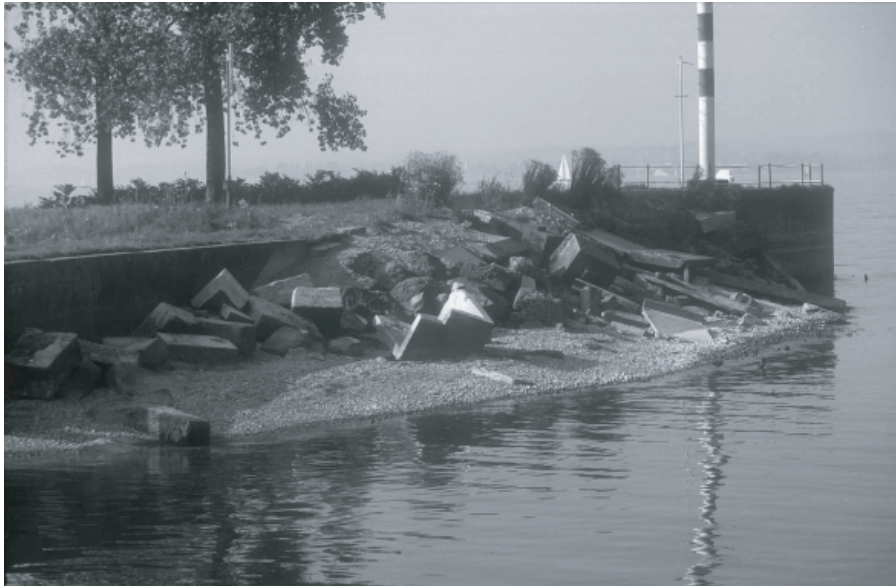
Fig. 4. Damaged shore fortifications on the eastern shore of Lake Constance near Bregenz.
